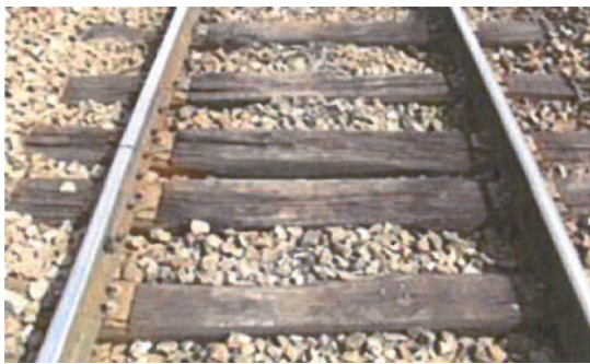
Illustration 5: Rails courts sur traverses bois
